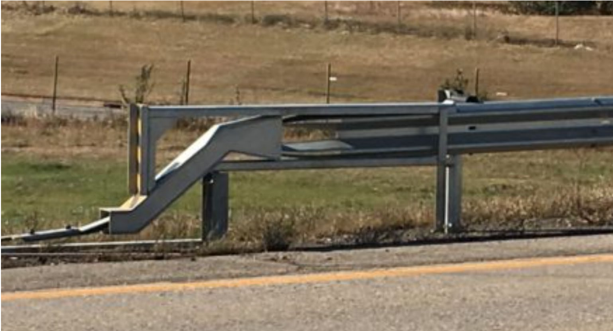
Correct Installation (Notice no bolt is visible at Post No.2)
