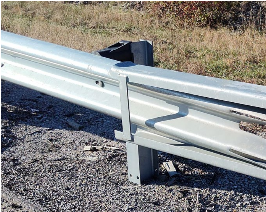
Incorrect Installation (Notice Bolt is visible and bolted through the rail at Post No.2)
